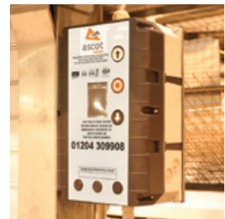
direct drive control panel
