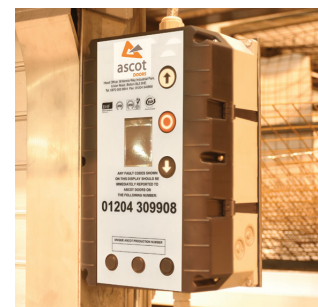
direct drive control panel
